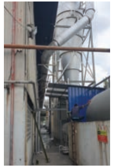
The new furnace for green fuel station.
